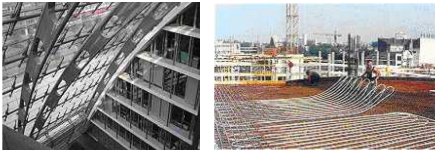
Figure 3.10 – Berliner Bogen: example of the building construction – double skin facade and floor slabs (left) where activating system of pipes was embedded (right) ( www.velta.de )
