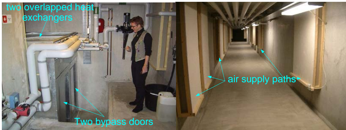
Figure 4.9. Air distribution duct of Mediå school (Left photo shows heat exchangers and “summer” doors. Right photo shows the supply air paths) (Tjelflaat 2002a).
