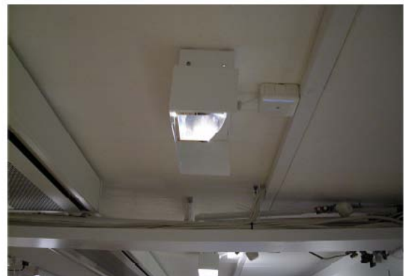
Figure 10-31. Lighting with Fortimo luminaire.
