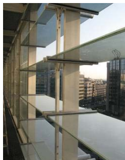
Figure 6-37. Louvres in horizontal position.
