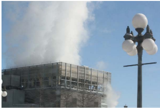
Figure 7.27: St. Paul District Energy Steam Turbine Cooling Tower - Winter.
