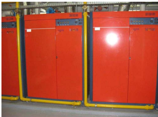
Figure 2-22: Hot water production plant
