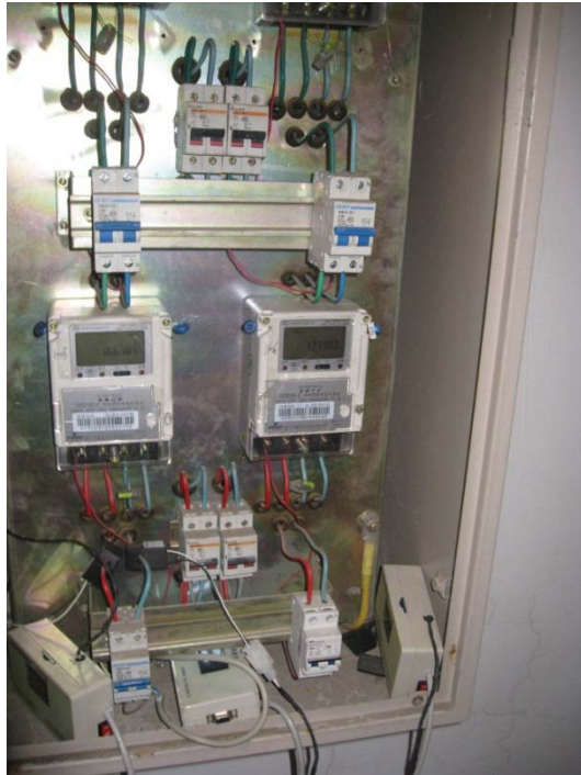
Power meters : Total scaled meter 1 and 2
