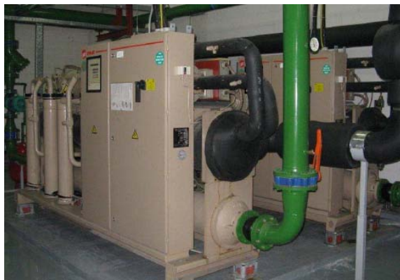
Figure 2-24: Water-cooled chilling package
