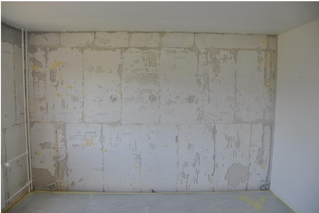
figure 13: View of gable wall after removing the internal insulation, to look for mould growth two years after installation. No mould growth was identified; however, the view shows that the insulation system did not fully bond to the existing wall. © AAU
